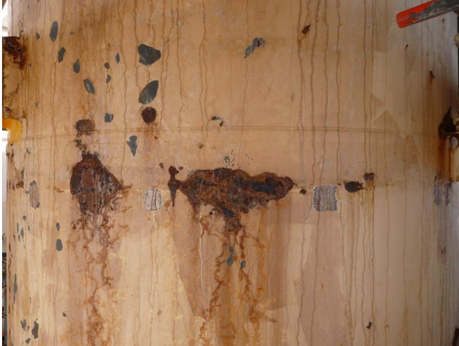
Corrosion under insulation (CUI)
