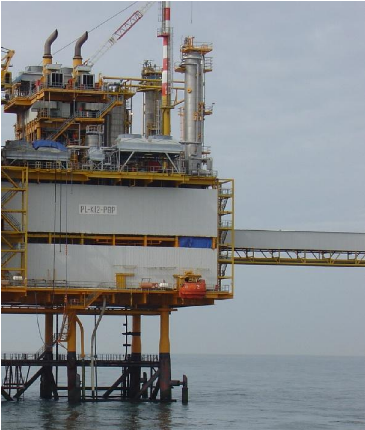
1151-B MDEA gas absorber (upper right tower)
